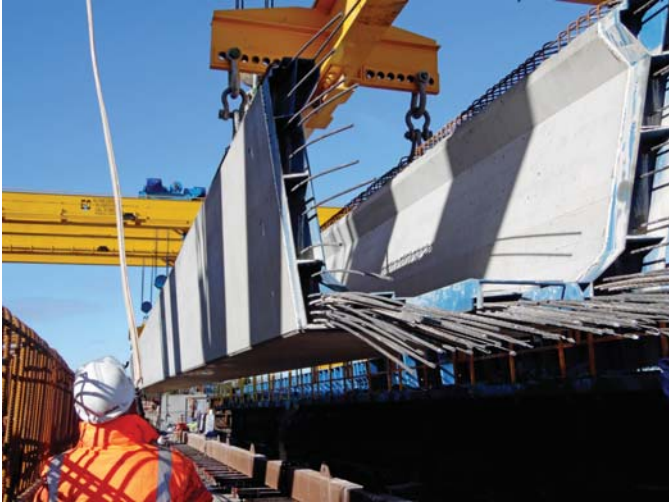
Above: The beams for the Raith interchange project were manufactured in steel formwork using a high-quality self-compacting concrete.
